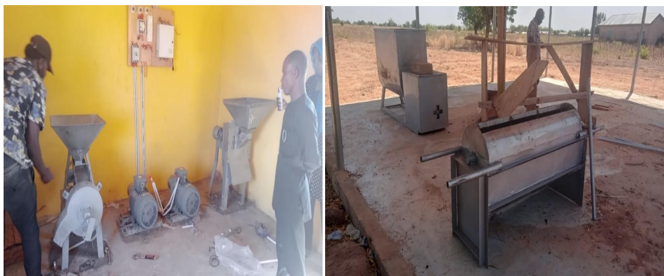
Figure 4.3 Installed equipment at the Zugu Shea Processing centre
